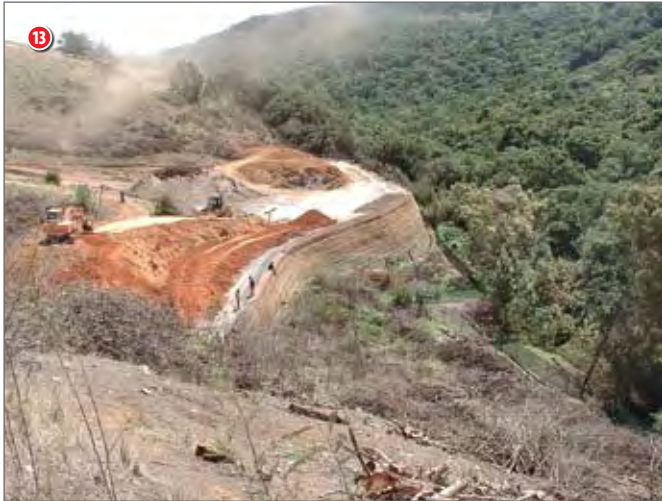
14 Aerial view of the GTM embankment at King Shaka International Airport with the embankment at approximately 50% of the final height
