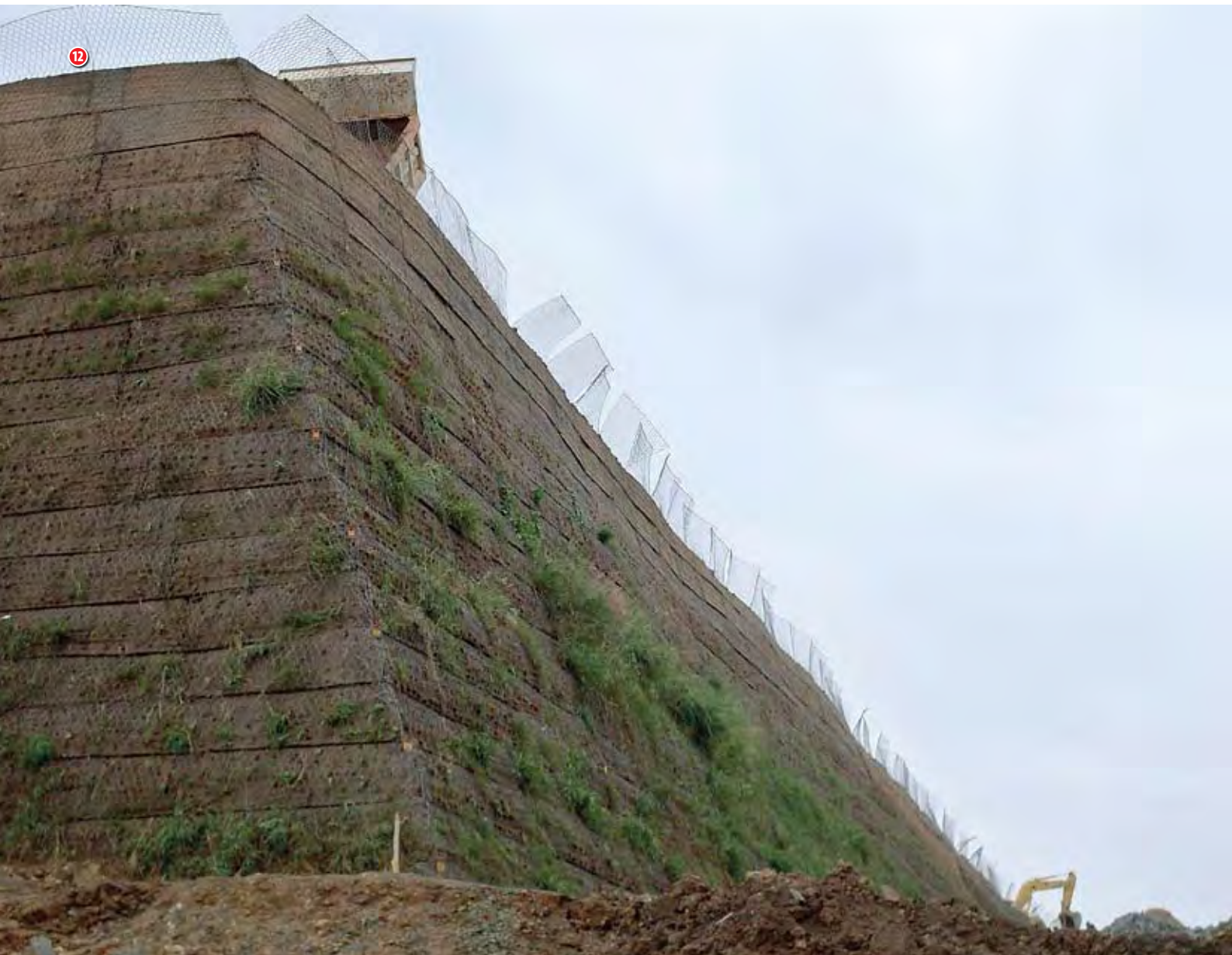
12 The GTM embankment at King Shaka International Airport at 80% of the final height, showing the initial growth of vegetation
